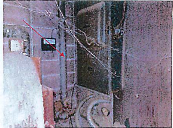
Photo #26 View of hard pipe insulation (HA-L) on the boiler piping throughout the building.
