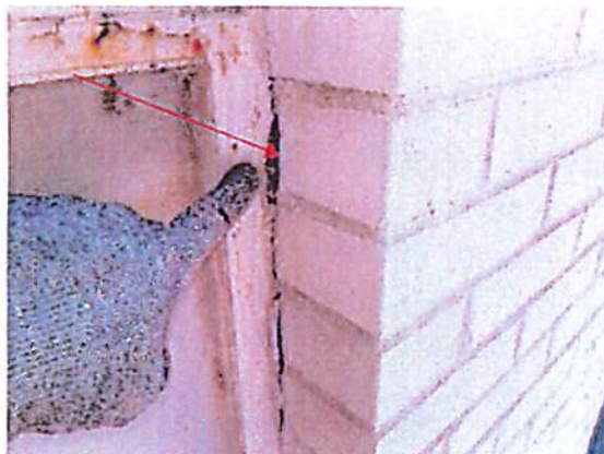
Photo #23 View of exterior door caulking (HA-H) on exterior windows throughout.
