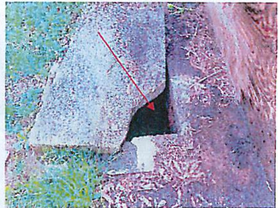
Photo #14 View of grease or septic tank located at the northern corner of the building.
