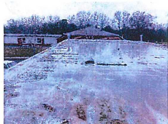
Photo #12 General view of the roof of the remainder of the building.
