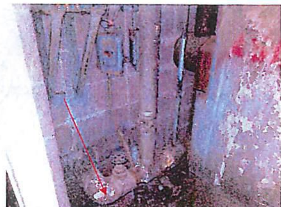
Photo #24 View of hard joints (HA-J) on boiler piping throughout the building.
