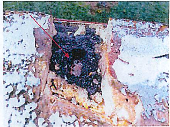
Photo #28 View of edge/penetration flashing (HA-N) under spray foam on the roof.
