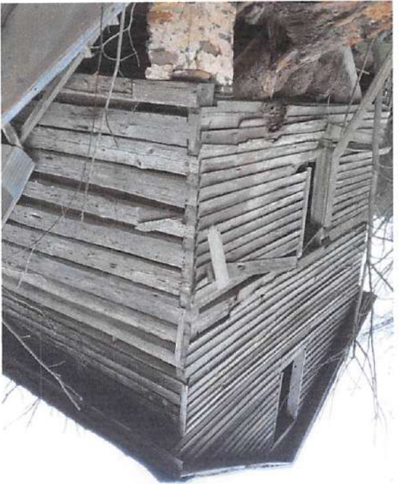
Log cabin near the Chauga River built in 1835. The exterior had been covered in siding which protected the logs.
