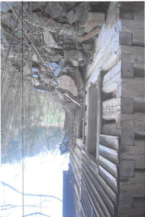
This photo shows the unusual Flat Notch and the collapsed rock chimney.
