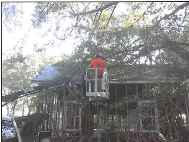
A huge "Thank You" to TreeSouth for clearing around our worksite in preparation of taking the roof off the main house.
