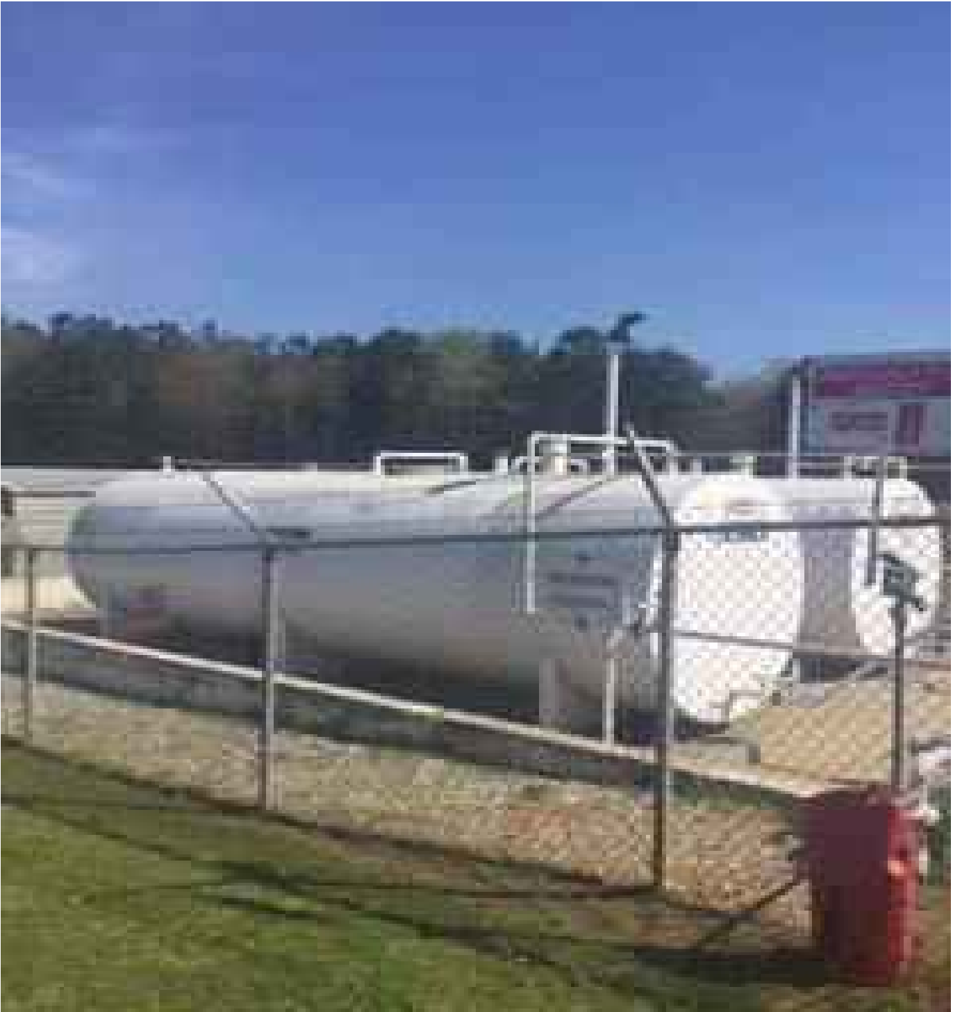
Fuel Farm and Containment Wall
