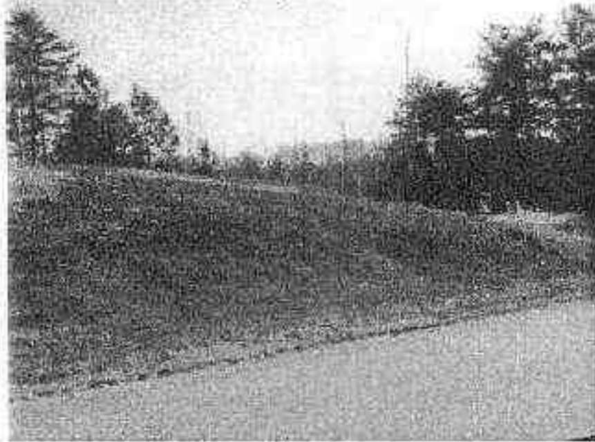
Photo 5: Stabilization issues at the intersection of Comet View Court and Twin View Drive.
