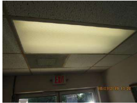
Lighting Brown Bldg..
