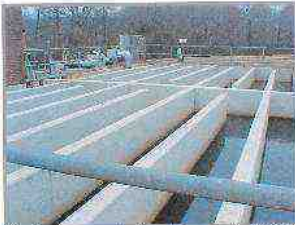
The chlorine contact chamber at Conners Creek WWTP provides disinfection for the wastewater.
