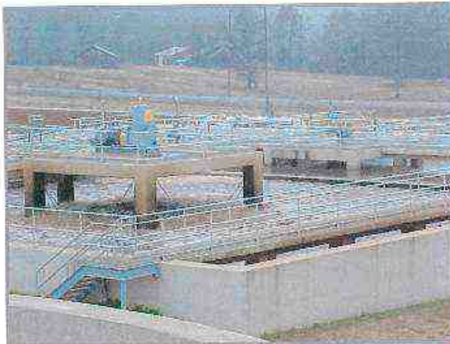
Rotators at Converse WWTP provide oxygen for the wastewater treatment process.
