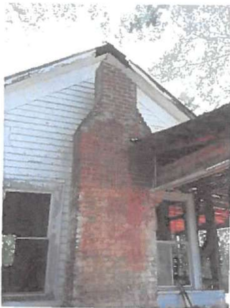
Photo of 1 (of 3) chimneys to be rebuilt. This photo was taken shortly after the dismantling began.
