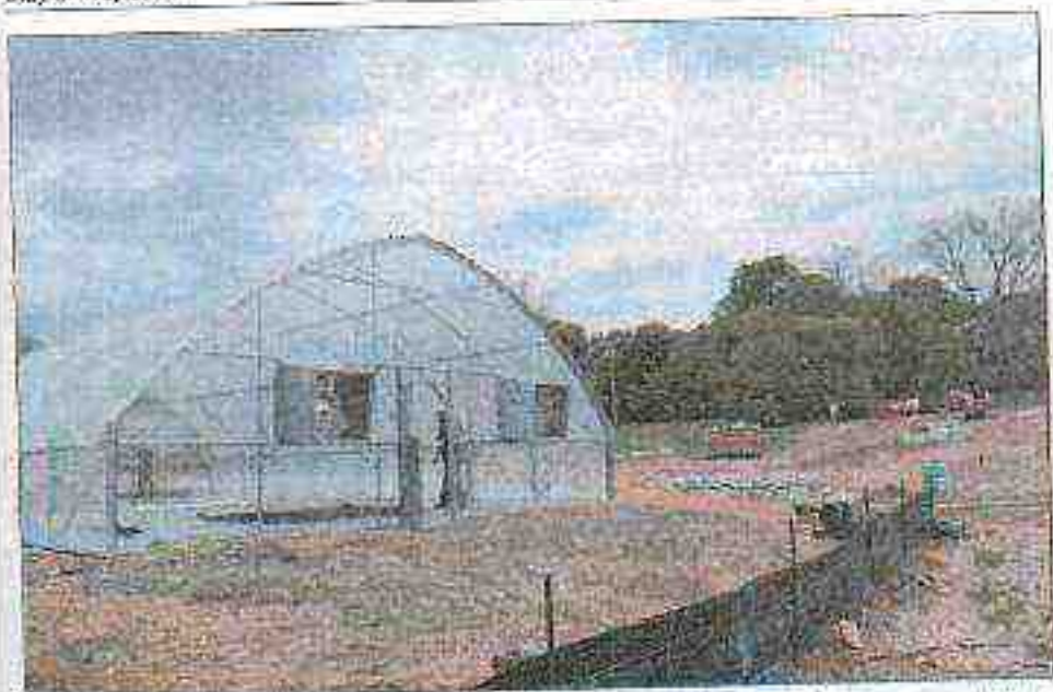
The Healthy Food Hub's greenhouse is the first structure of several to go into the space as part of an effort to revitalize Spartanburg's Northside community. (Photo: Ashley Baccinino)
