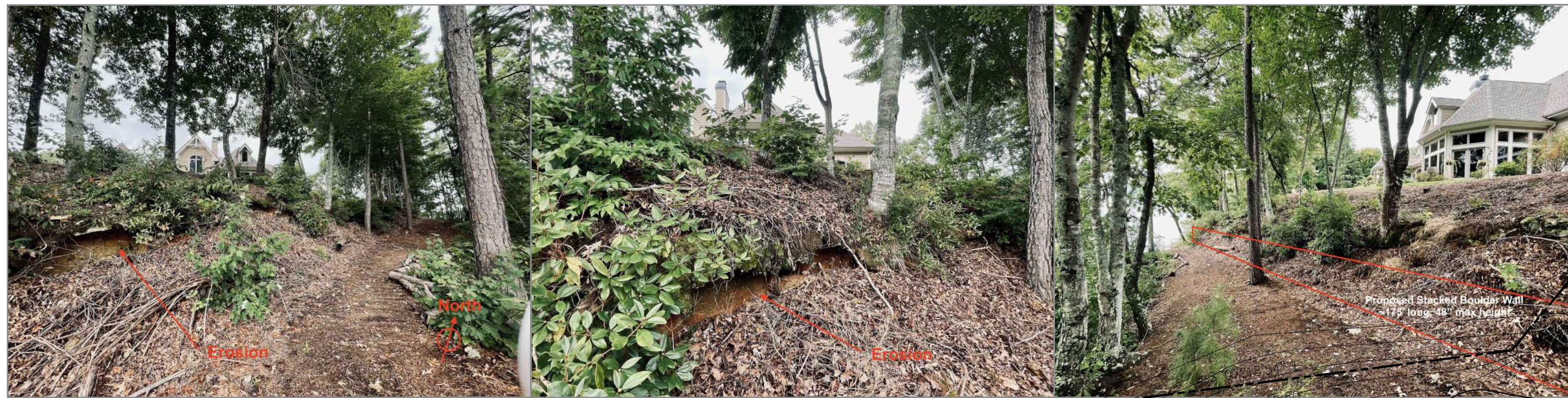
VIEWS OF EXISTING ERODING LAKESIDE BANK. +/- 175' LONG x 4' TALL (MAX) BOULDER RETAINING WALL TO BE INSTALLED TO STABILIZE BANK.
