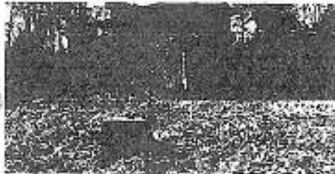
Mulch and backfill on left side of Slotter foundation facing Stevenson home.jpg
