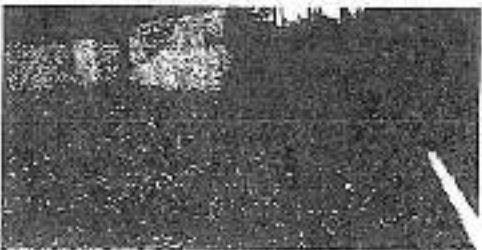
Silt fence looking up from retaining wall between Johnson and Slotter lots.jpg
