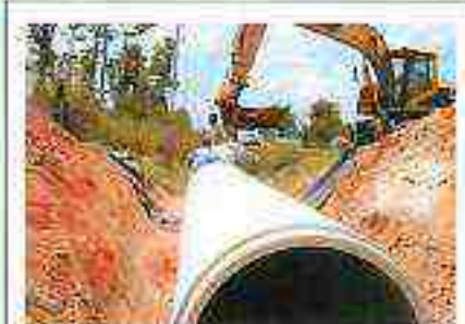
ACOG Grant Services routinely assists communities with grants related to infrastructure repair and improvement.
