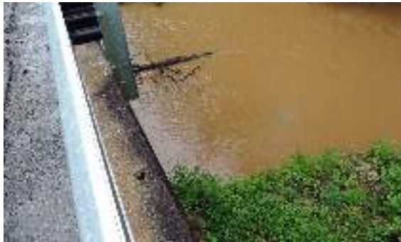
Debris upstream of Burns Mill Bridge
