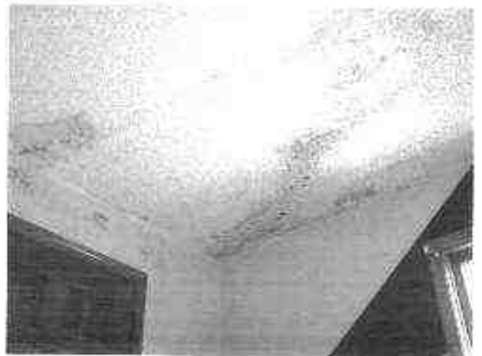
Examples of Disrepair/Damage to CAP house on Airport Property
