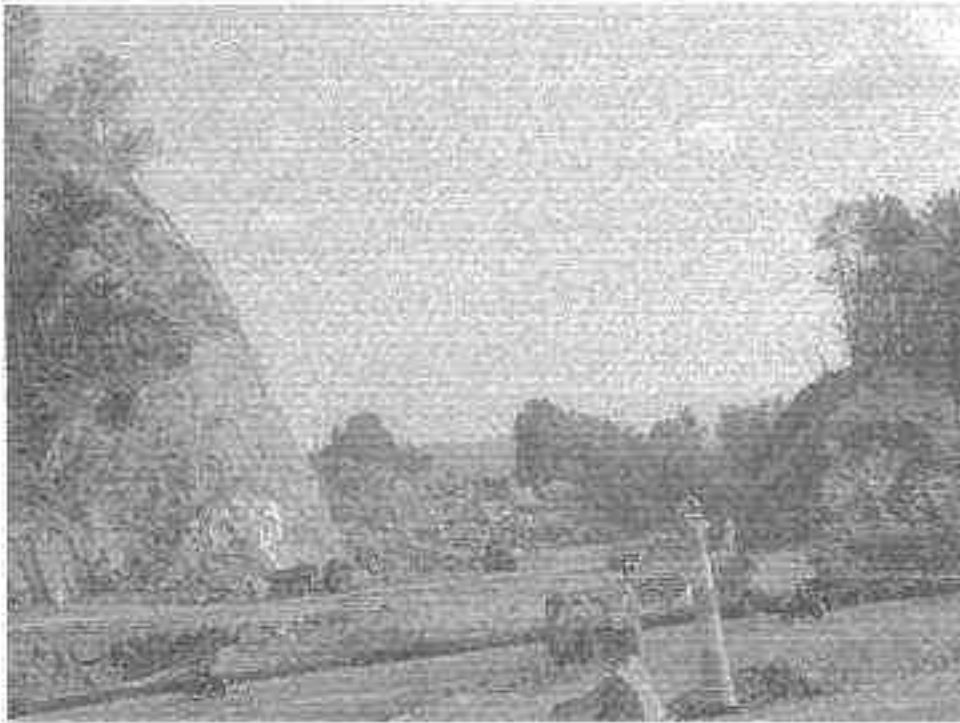
A simple four-laning project on Highway 321 between Lenoir and Blowing Rock in North Carolina. Note the size of the yellow construction dump truck, dwarfed by the project. An interstate highway requires 3 times this width.
